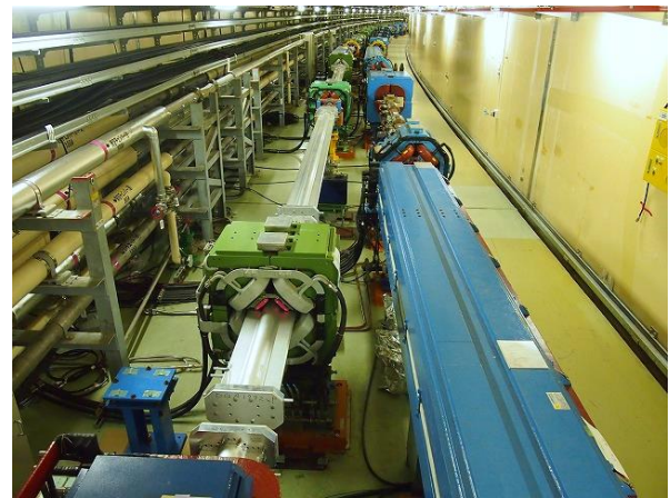
Figure 3: An arc section of SuperKEKB. The right hand side ring is HER. Left is LER. New cooling water pipes are seen along the outside tunnel wall.
